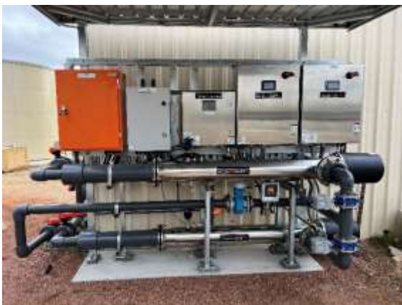
New UV Filter System at Isisford WTP.
