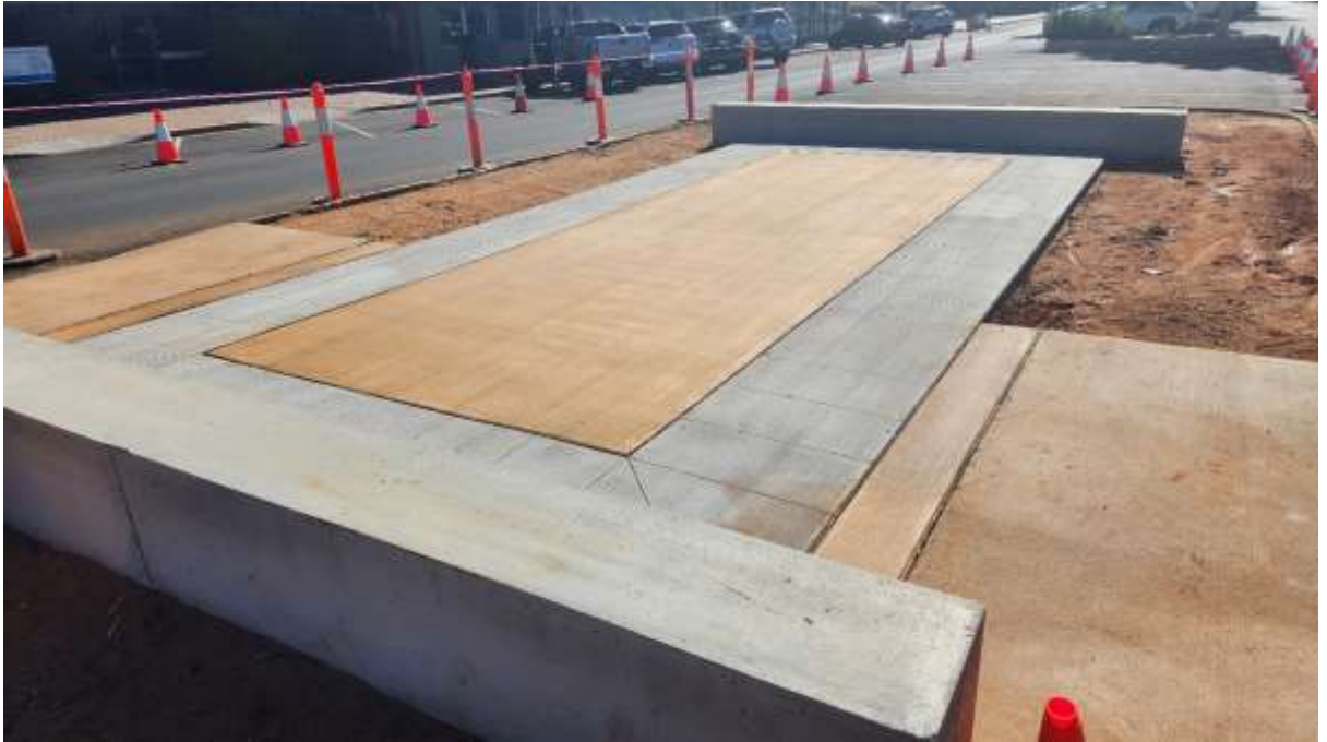
Pictured above: Eagle Street centre median, awaiting flagstone walls and garden installation.
