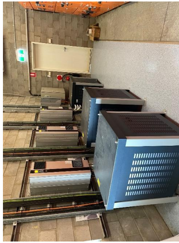
Photo 4: Water Treatment Plant – no noise signage in pump room
