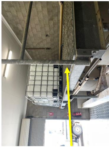
Photo 1: Water Treatment Plant – Coagulant rack guarding
