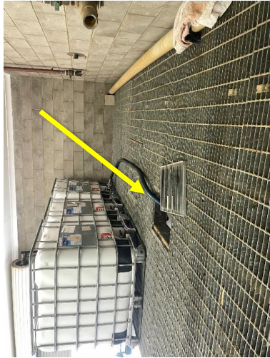
Photo 2: Water Treatment Plant – Coagulant rack platform
