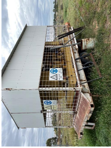
Photo 3: Water Treatment Plant – Generator
