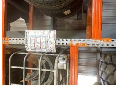
Photo 6: Workshop – Racking audit not current.
